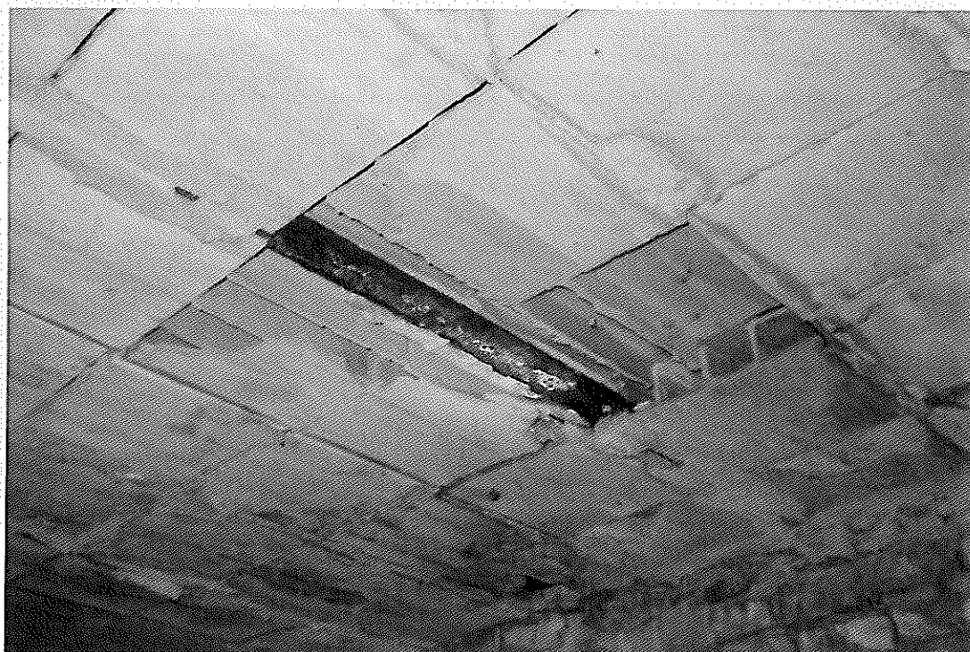
4 – PIANO INTERRATO : TRAVE IN FERRO ARRUGGINITA
